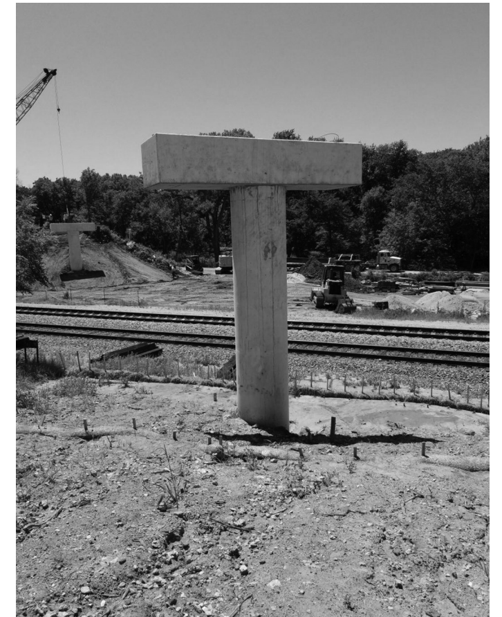
Pier for the new Rock Island—Jamaica North Trail Bridge Image courtesy of Lincoln Parks & Recreation Department
