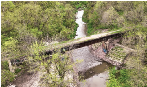
An aerial photograph of the Rock Island Bridge over Salt Creek prior to construction.
